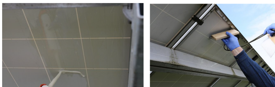
FIGURE 4 Application of the silicone sealant in the field without dismantling the modules
